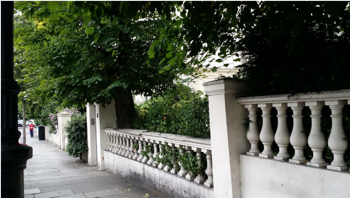
Length of wall to be replaced including two piers to the north.
